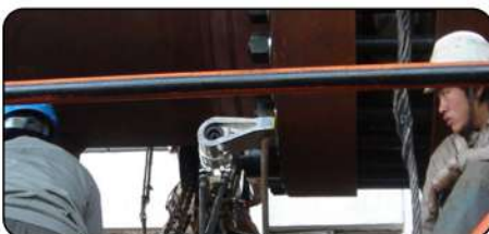
Refinery Pressure Vessel Bolt Preload
