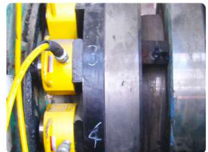
Synchronous separation for repairing the roller press and decelerator in the cement plant
