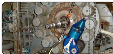
Removal of inspection bolts for high pressure feed water pump in thermal power plant
