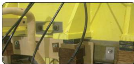
Large transformer assembly and compression
