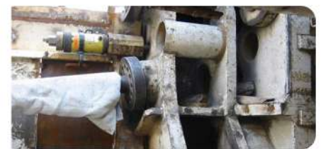
Shield machine maintenance application
