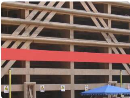
Synchronous lifting and maintenance of herringbone door
